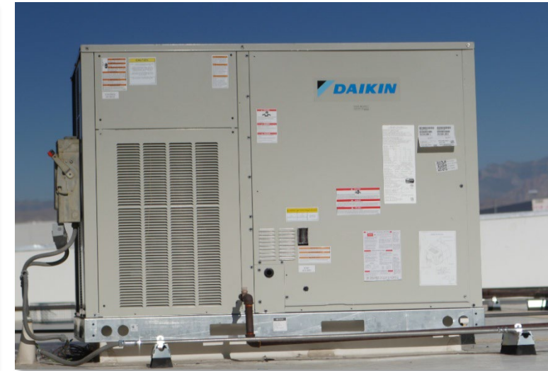
Daikin unit installed on original roof curb without a curb adapter
